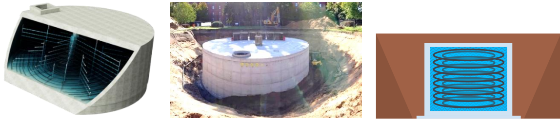
Fig. 1: Concrete tank ice store concept. Left: 3D graphic providing an internal view of the ice store, showing the heat exchanger coils and their mounting (LTTT, 2025). Middle: photograph taken during the construction phase (Krug, 2019). Right: simplified schematic.
