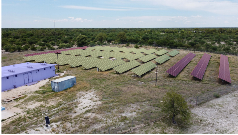
Fig. 1: Aerial view of the existing Tsumkwe hybrid mini-grid: The 202 kW p (2012, yellow overlay) and 102 kW p (2016, red overlay) ground-mounted PV fields and the building housing the battery storage (blue overlay). Source: Institute of new Energy Systems (InES), TH Ingolstadt. Edited for annotation and to remove extraneous foreground elements.
