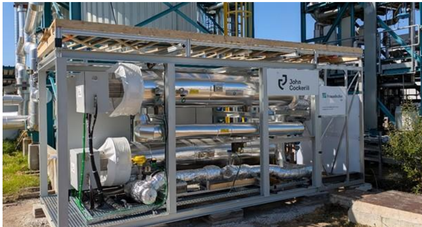
Fig. 1: The power-to-heat unit prototype with a two-stage electric heater integrated into the test loop with two tank TES.
