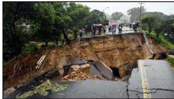
Damage of roads and electric poles
