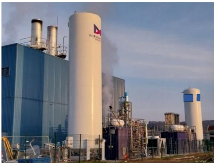
Figure 1 : Carbon purification and liquefaction unit installed in Villers-Saint-Paul plant
