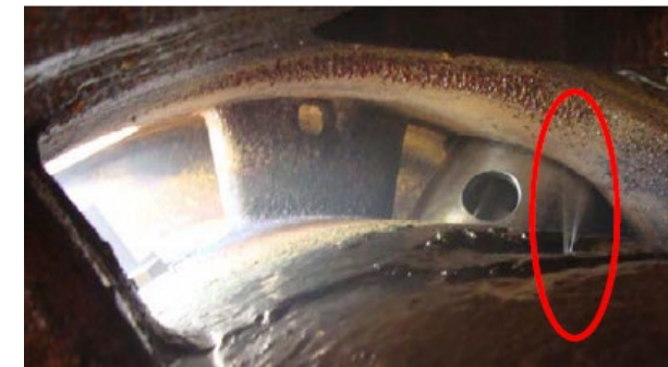
3rd stage compressor (14/01/2010)
