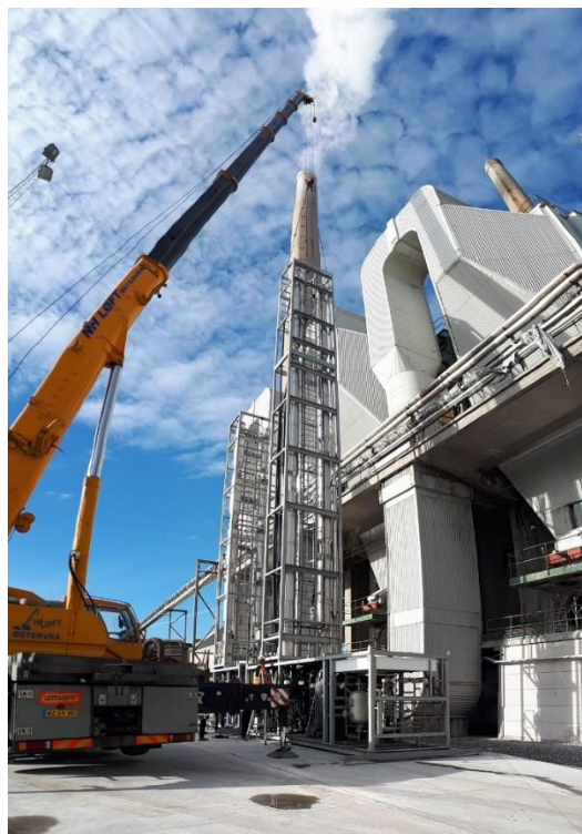
Figure 1: CO 2 capture pilot plant installation at Aalborg Portland
