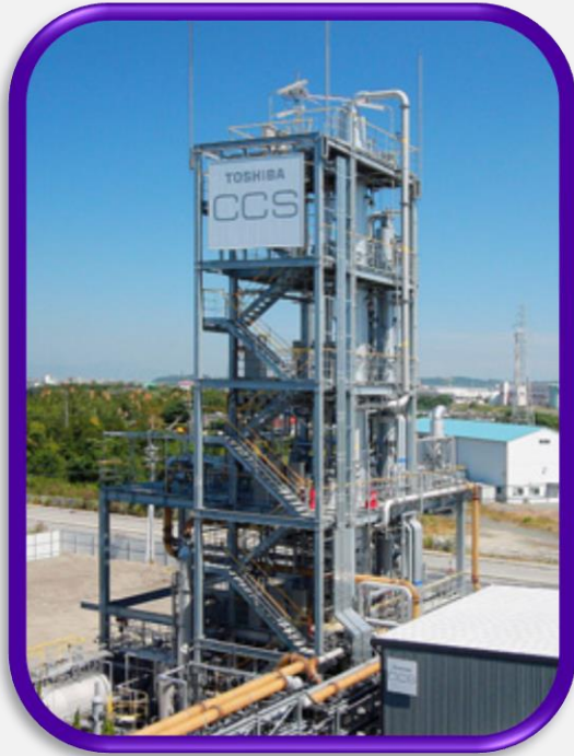
Mikawa Pilot Plant, 10 tonnes/day, (Toshiba 2009)
