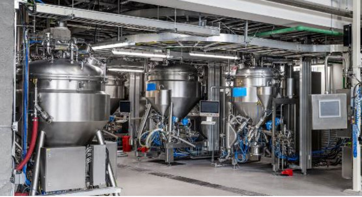
Sorbent Slurry Room
