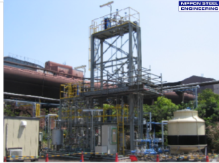
1t/d test plant
