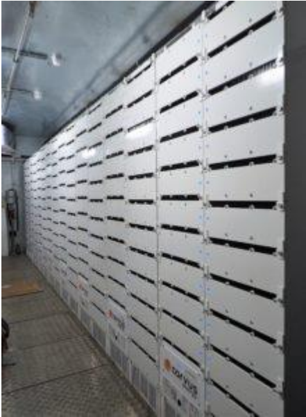
Energy storage system (ESS)
