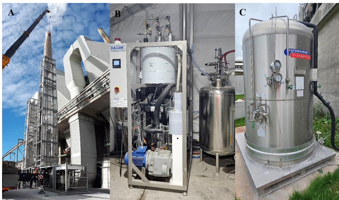
Figure 1 Overview of the process equipment included in the test unit located at Aalborg Portland. A) CO 2 capture pilot plant, B) CO 2 liquefaction, and C) temporary CO 2 storage.
