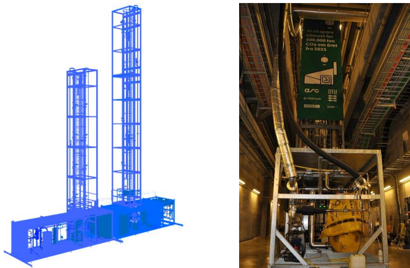
Figure 1: Mobile capture plant. (a) 3D Drawing of the pilot plant (b) The pilot plant located at Amger Bakke, a WtE facility in Copenhagen, Denmark. (Vinjarapu, Neerup, Larsen, Villadsen, et al., 2024)
