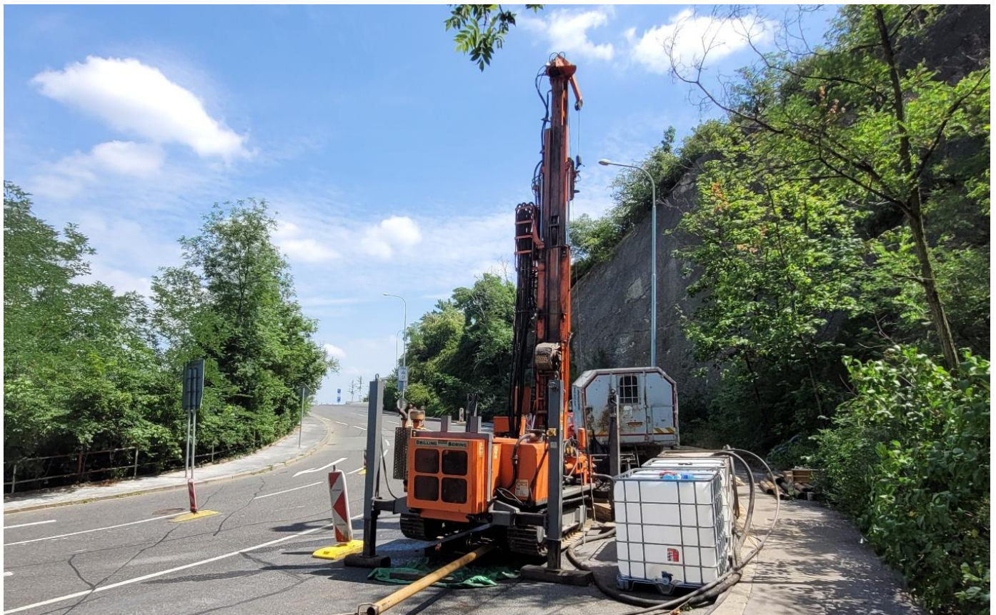
Figure 4: Execution of exploratory borehole J1 in the serpentines of Barrandovská Street in Prague (June 2024).
