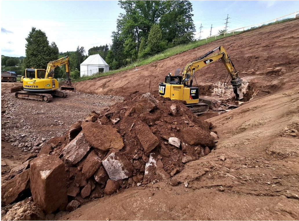
Figure 7: Excavation works in the central trench area – direct transition from Quaternary cover to bedrock
