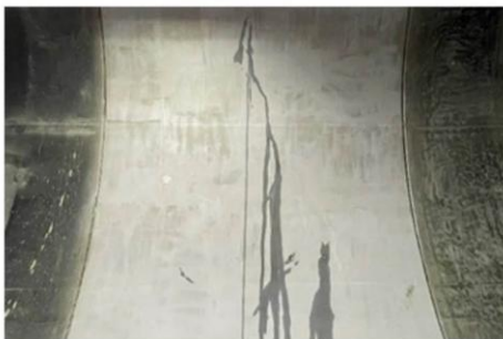
Figure 16: Cracking of the UHPFRC inner lining after casting
