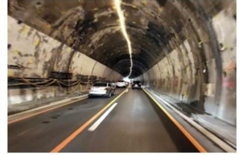
Figure 24: Tunnel prior to renovation, showing waterproofing defects
