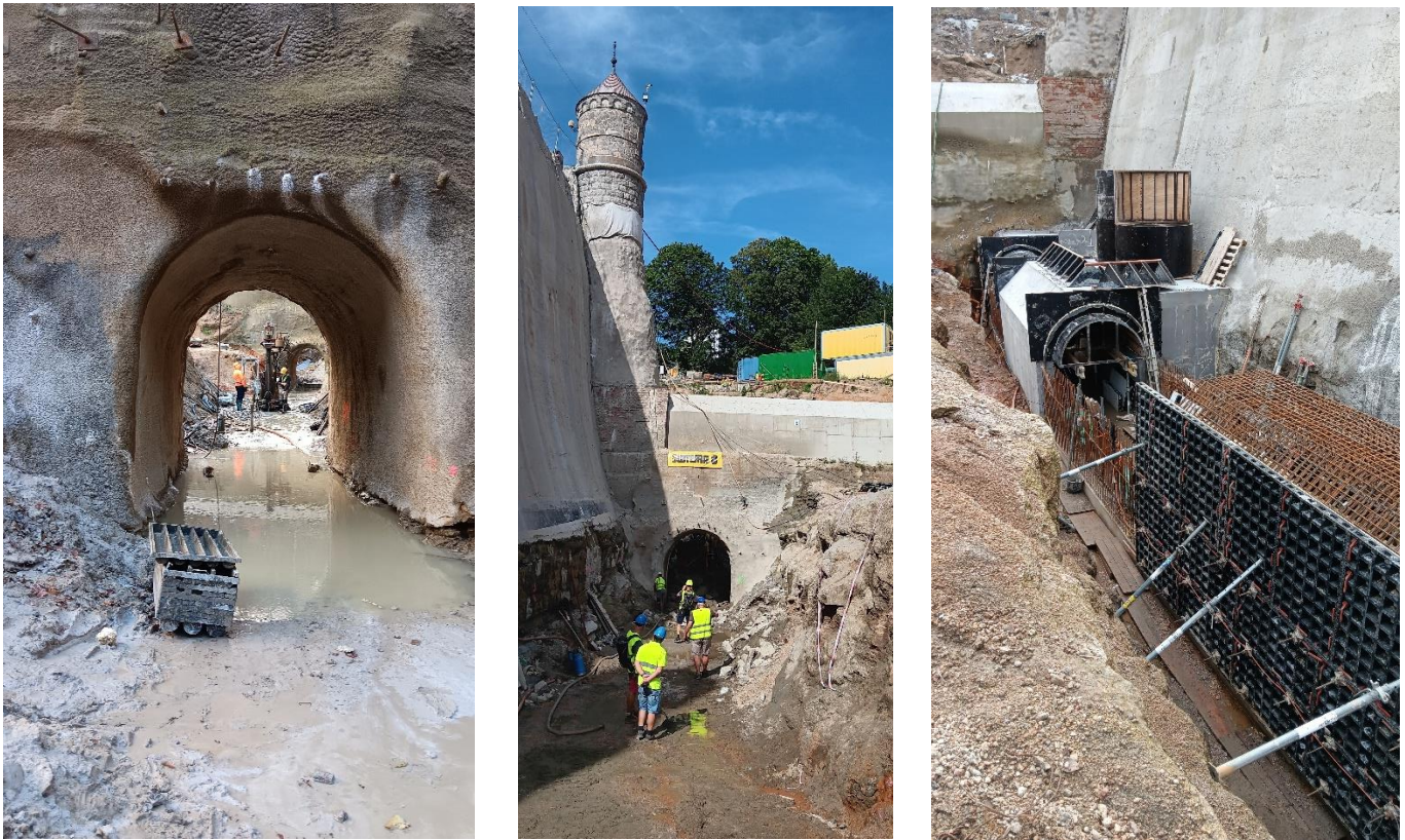
Fig. 4 a 5 View of both sections of excavations in the axis of the future gallery. Fig. 6 Gallery lining concreting
