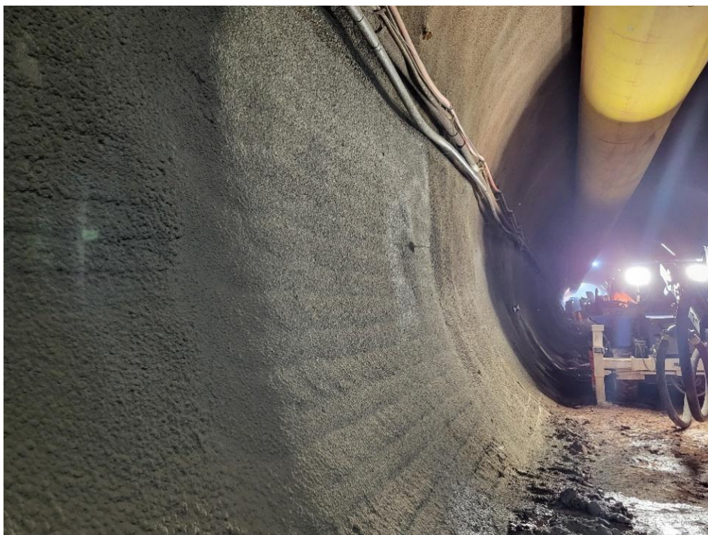
Figure 4: Scan of sprayed surface plotted against the set profile (the green areas at the shoulder were not intended to be sprayed)
