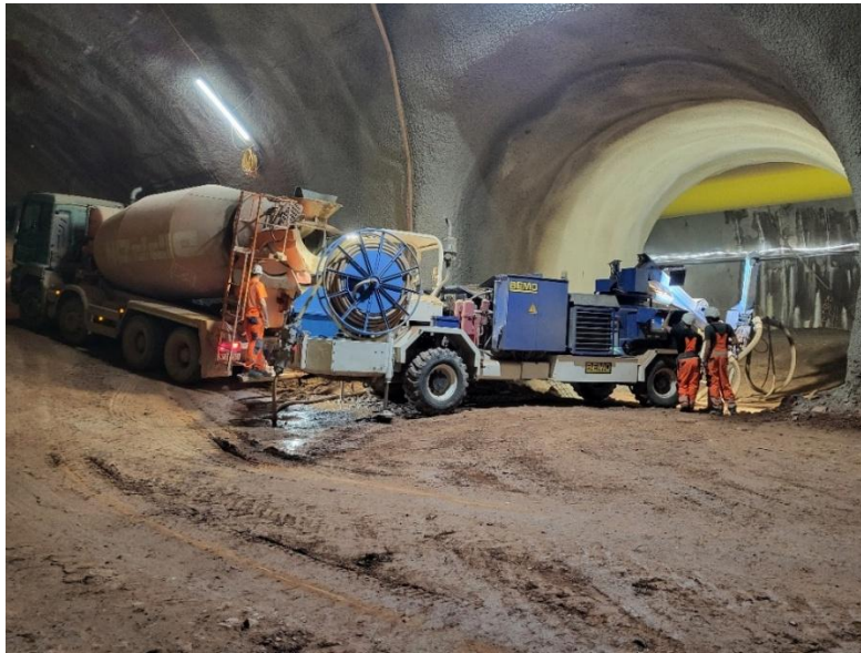
Figure 9: position of spray-robot in cross passage ready to start spraying the first section on the opposite side
