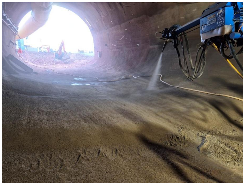
Figure 16: spraying the invert; noticeable is the gap right in the tunnel axis of the invert which has to be eliminated
