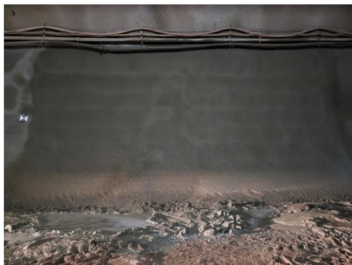
Figure 8: three block joints (the first located next to the surveying target) after execution of the final layer without visible herringbone pattern and with smoothly executed transitions
