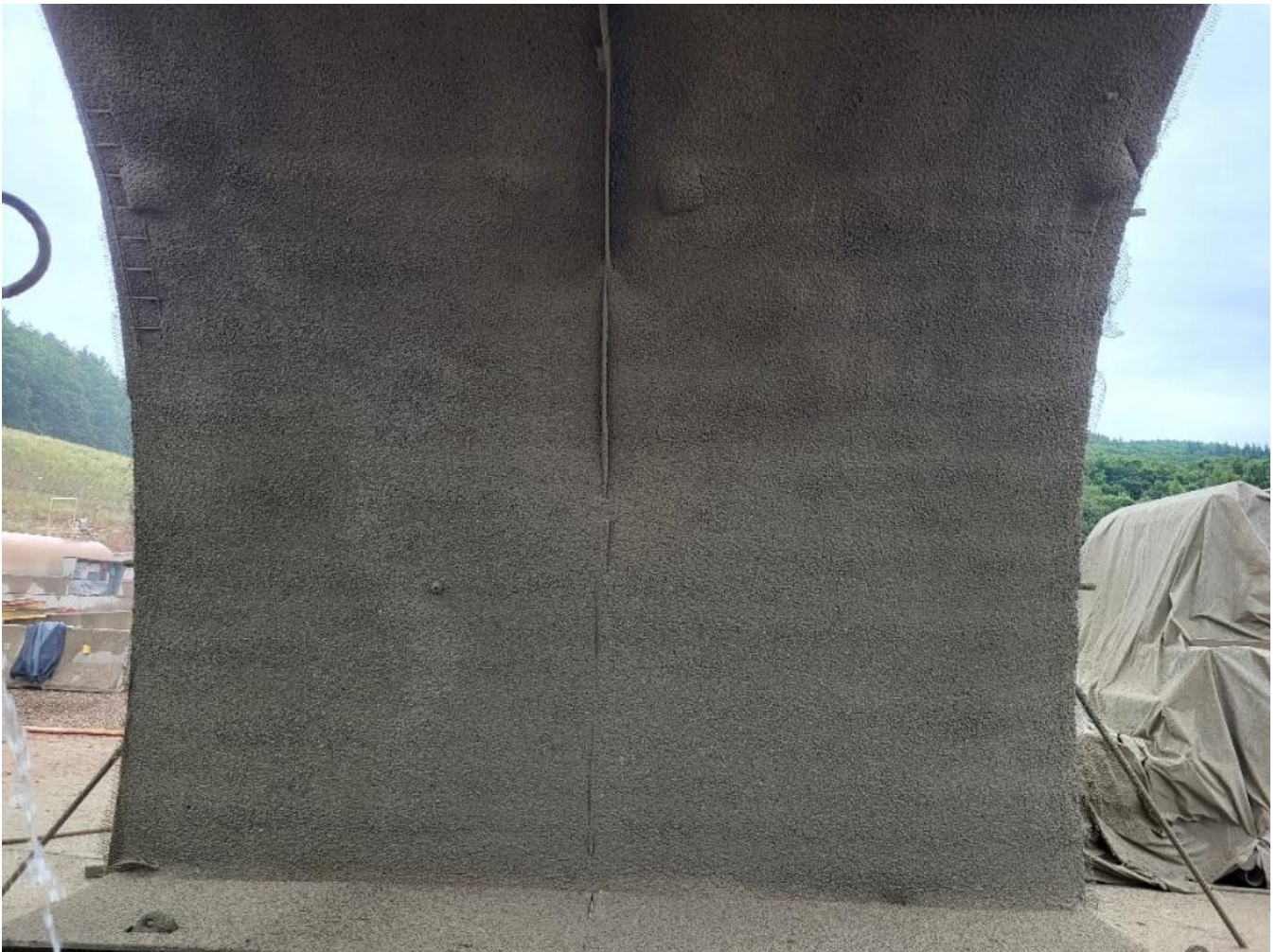
Figure 2: spray surface result at mock-up at Holsteintunnel Germany; a bolt head on the left part of the structure shows perfectly smooth overspray (the bolt plates at the shoulder of the structure were not intended to be sprayed in entirety)
