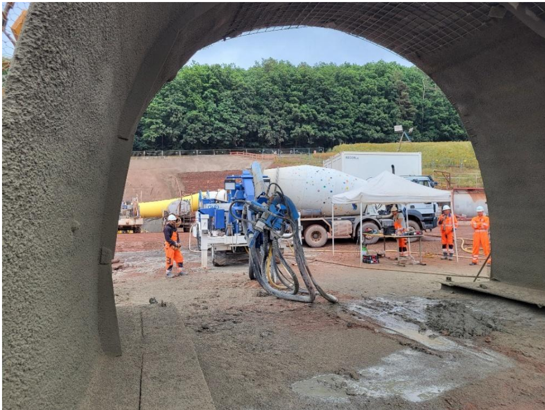
Figure 1: mock-up at Holsteintunnel Germany; control IT set-up in background right to the sprayer
