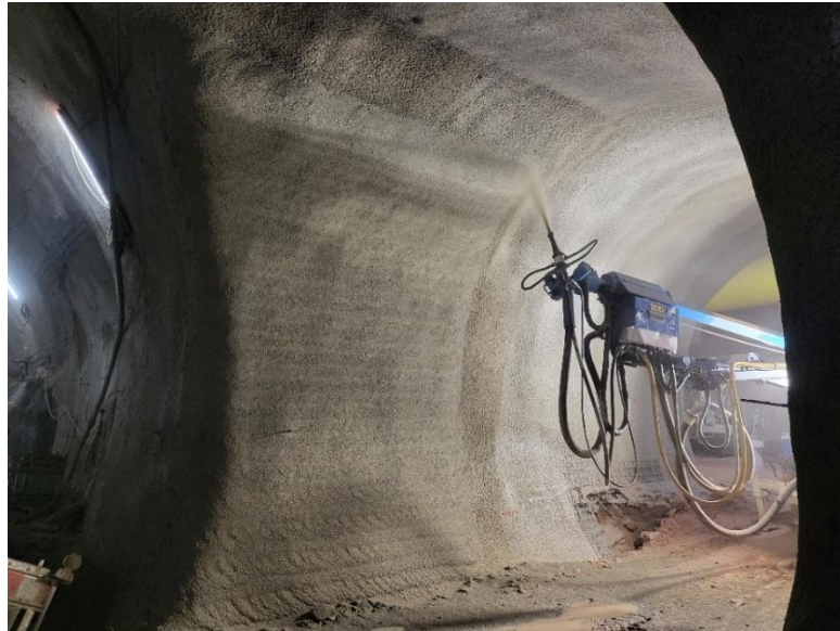
Figure 11: spraying the geometry layer of the intersection part of the cross passage and main tunnel; see the rebound covering the invert
