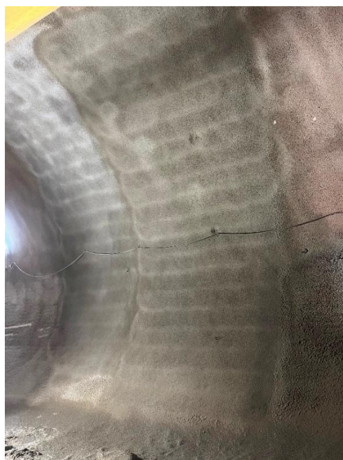
Figure 14: finished two blocks with geometry layer from invert and sidewall and final layer from invert to the crown centreline close to the ducting
