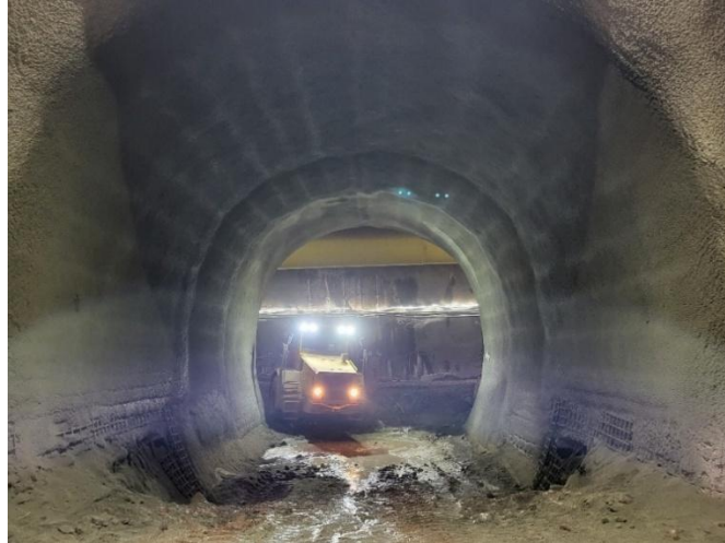
Figure 13: optical appearance of the completed cross passage; the horizontal lines are unavoidable due to the automated process which does not quite allow human style pattern and has to be accepted
