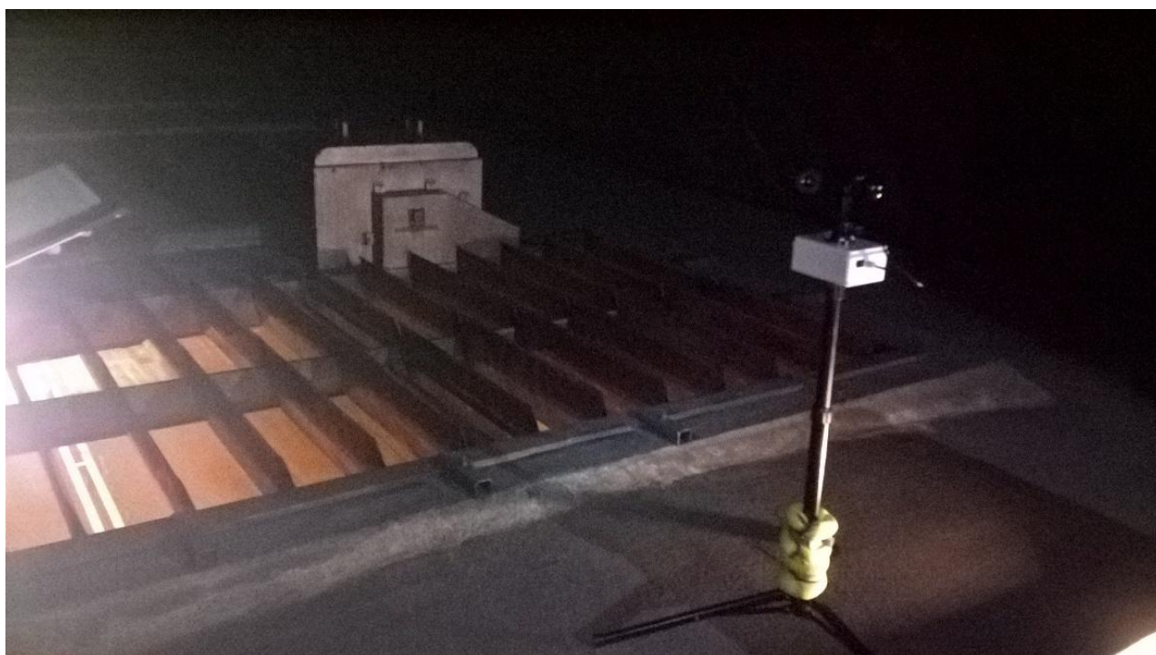
Figure 7: Anemometer in the ventilation duct of Branisko tunnel
