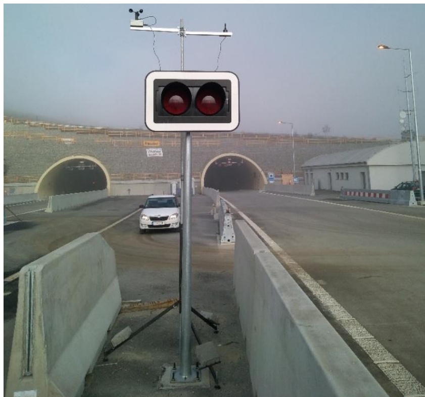
Figure 6: Anemometer with potentiometric wind-vane at the Ovčiarsko tunnel portal
