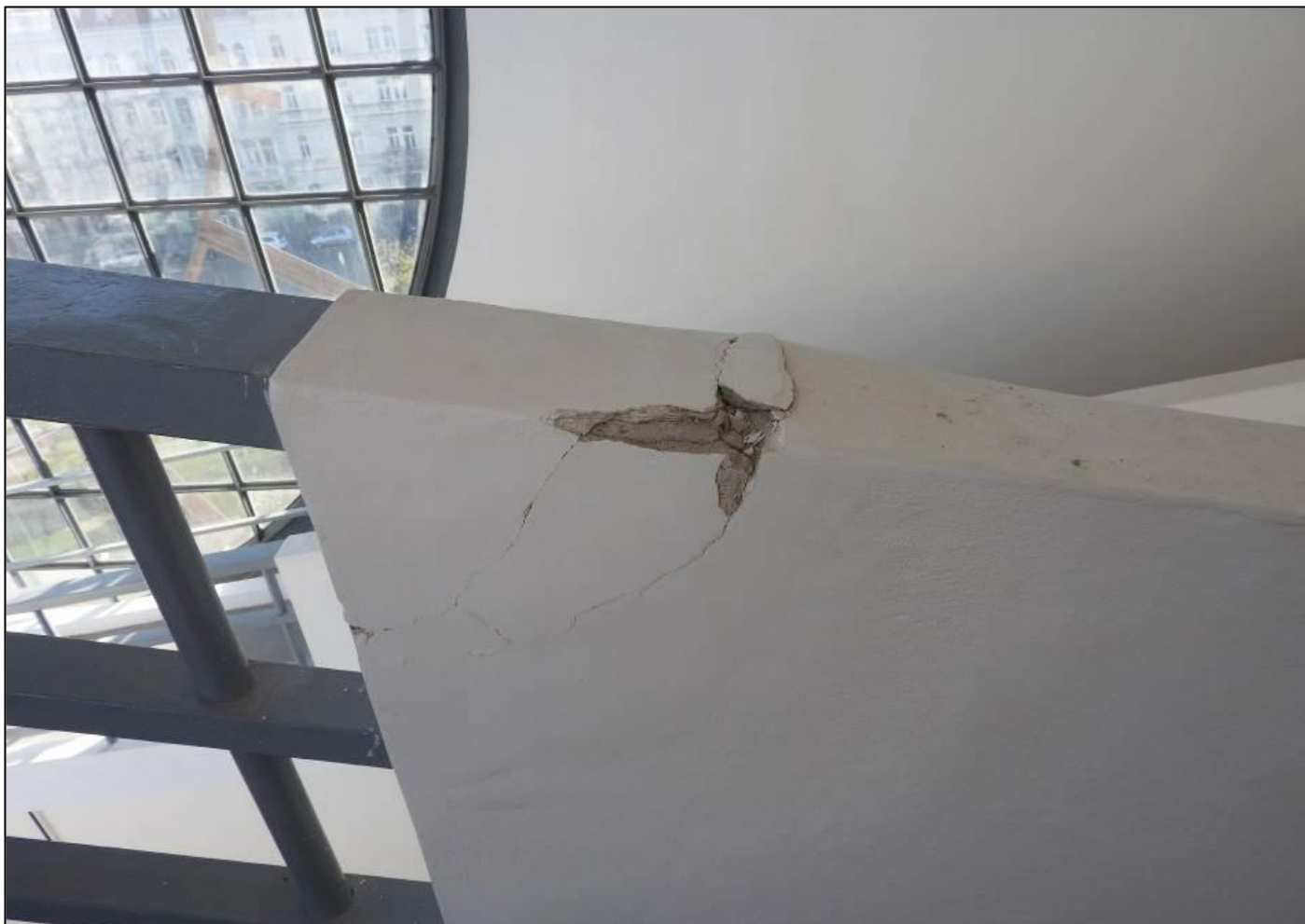
Figure 8: Damage at the point of attachment of the ramp railing due to temperature
