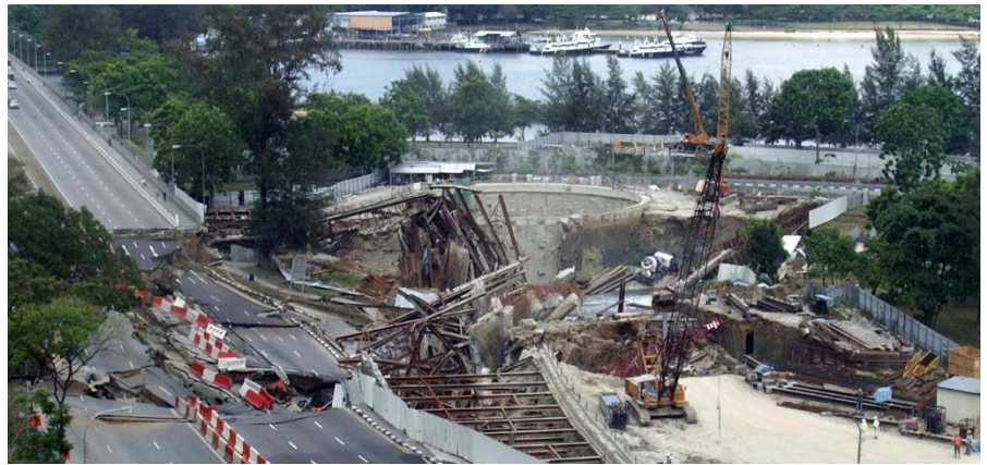
Figure 3: Collapse of metro construction pit due to buckling of struts in Singapore 2004 (Source: Hee Yang Ng, Structure Magazine 2021)
