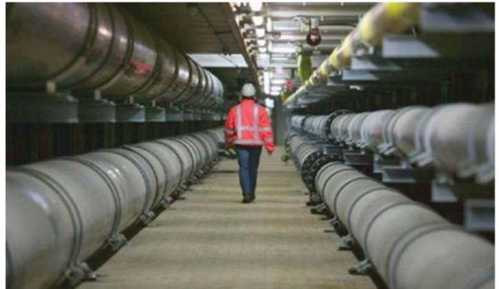
Figure 4 Utilidor in Amsterdam carries multiple utility lines SOURCE: Courtesy H. Admiraal.
