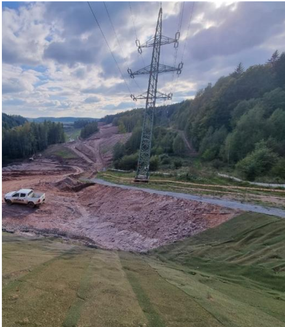
Figure 5: View of the VHV pylon from the crest of the excavation slope
