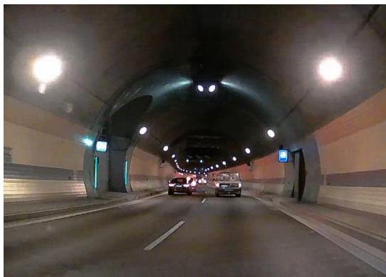
Figure 2: Example of the installation of green dynamic strip lights in TKB
