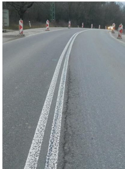
Figure 5: Location of cracks on the surface of road I/17.
