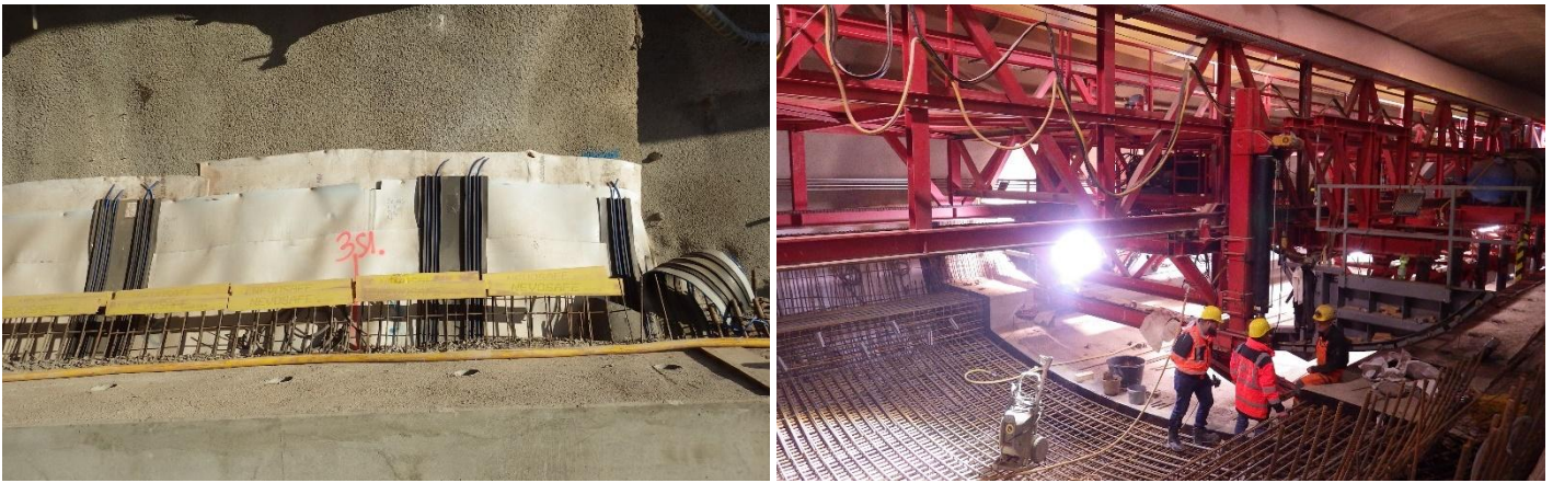
Figure 15: Sealing bands at transition between mined and cut-and-cover section, Figure 16: Invert concreting operations.
