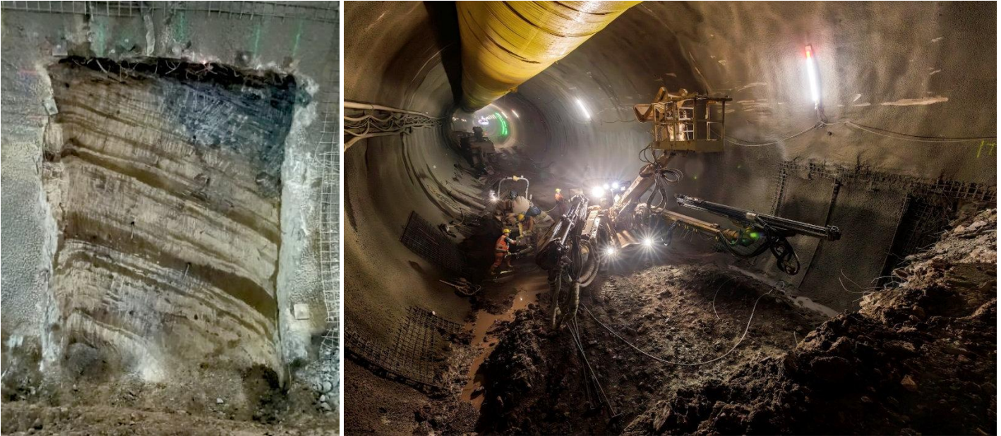
Figure 12: Excavation niche at geological transition zone, Figure 13: Bench excavation near cross-passage zone.
