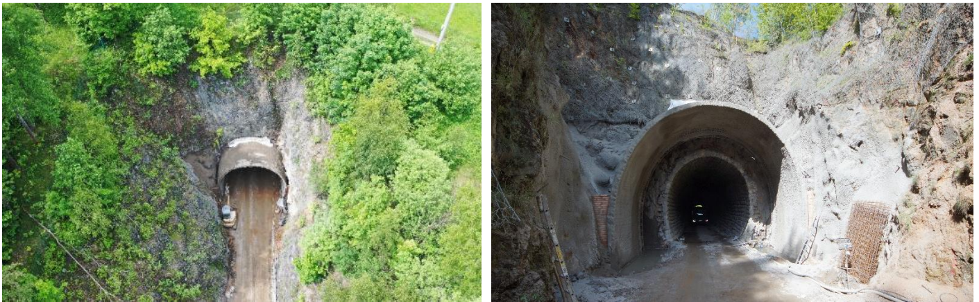
Fig. 16 Cramped space conditions at the tunnel portal in a deep rock cut
