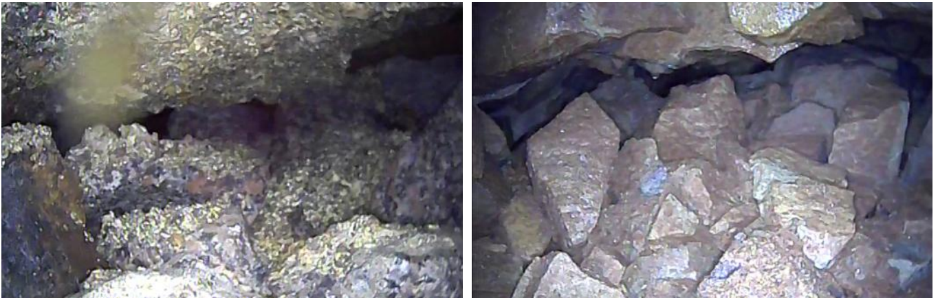
Fig. 14 Cavities captured by the camera behind the original tunnel lining
