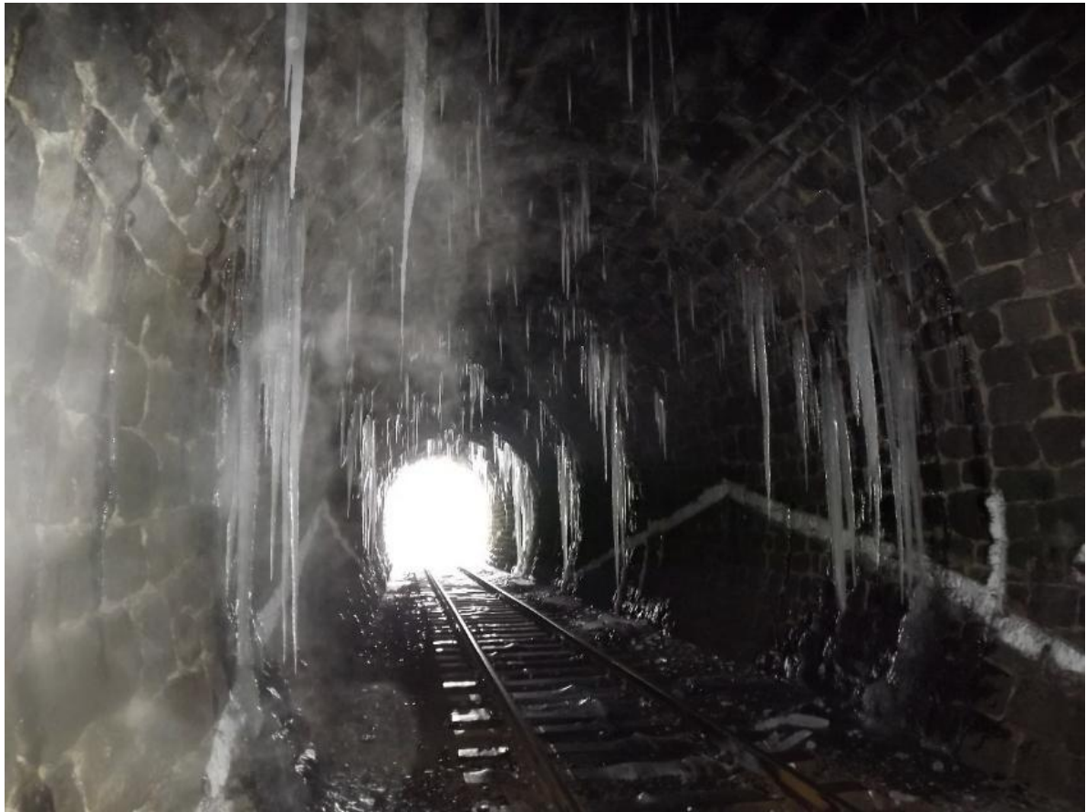
Figure 5 Massive icing of the tunnel due to groundwater seepage
