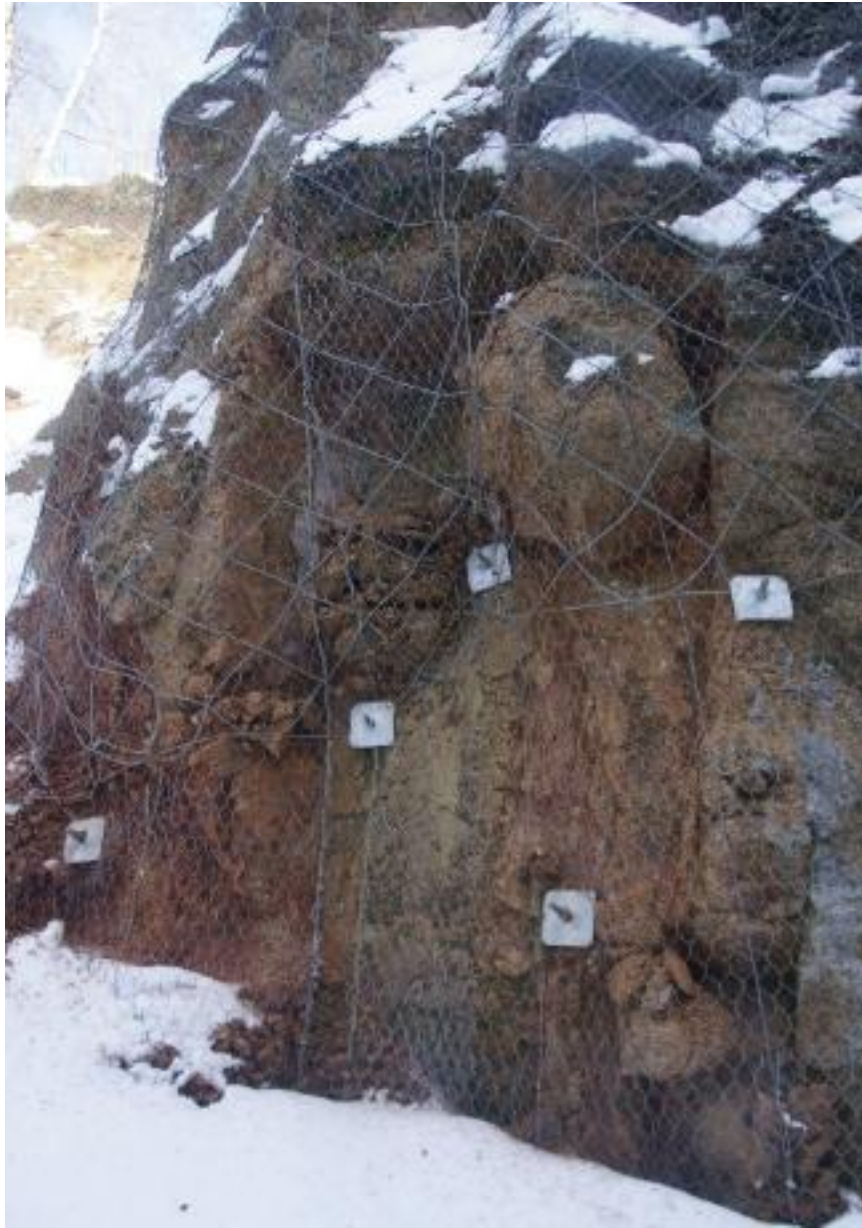
Figure 2 Rock block caught in a high-strength net on the side of the rock cut
