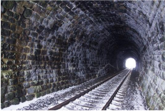
Figure 3 Condition of the brickwork during the dry season
