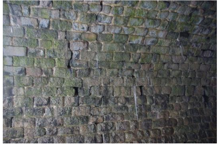
Figure 4 Vertical cracks in the lining
