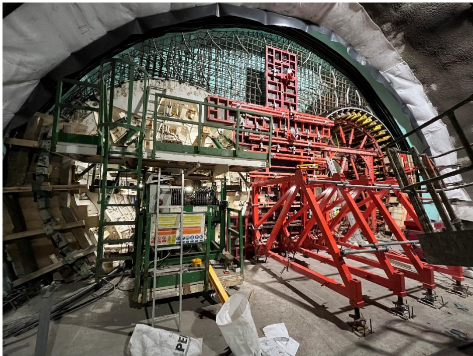
Figure 8- Formwork for the front wall of the junction to the C-D connection
