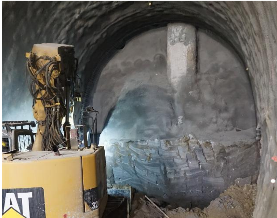
Figure 6: SEM excavation encountering the foundation of a high mast lighting pole.
