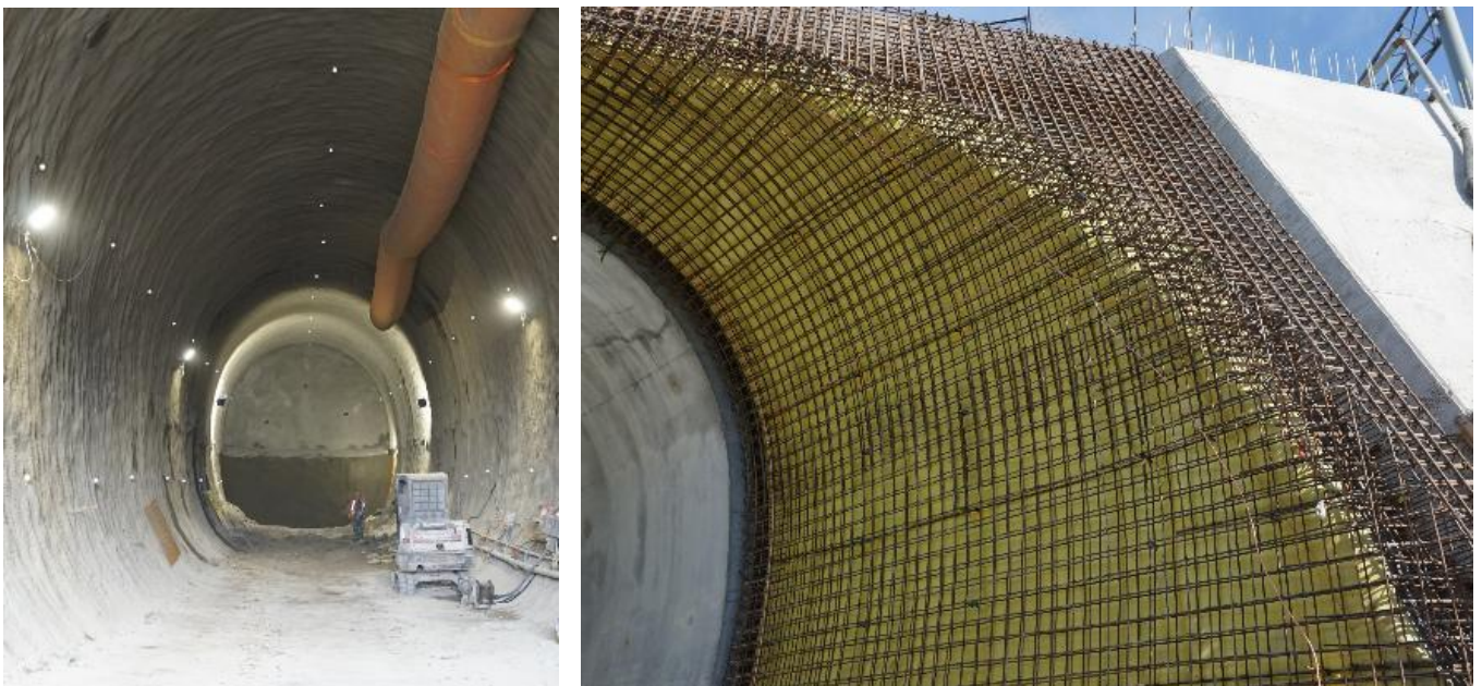
Figure 5: Initial shotcrete lining (left) and construction of the final support at the portal.
