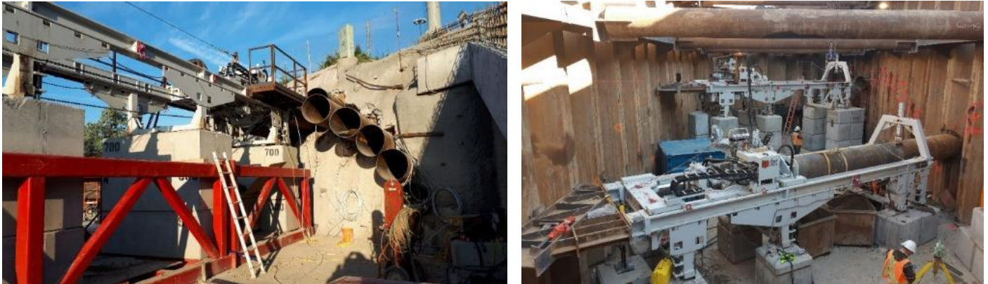
Figure 4: Installation of 813mm pre-support pipes from the portal (left) and the intermediate shaft (right).
