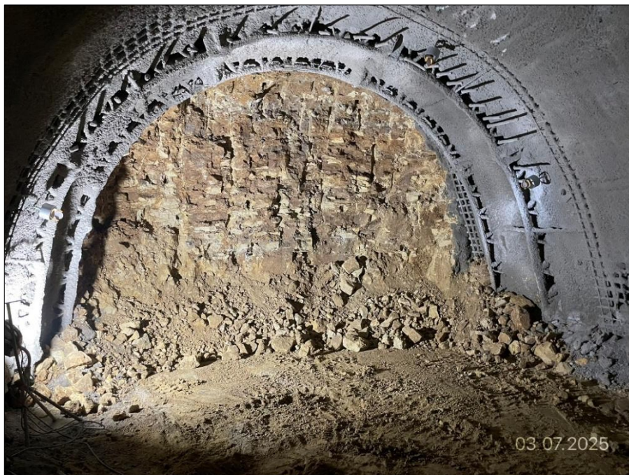
Fig. 6 Unsupported tunnel face of the top heading in variably weathered marlstone during excavation from the Š8 shaft towards the TK7 shaft (photo by the author)
