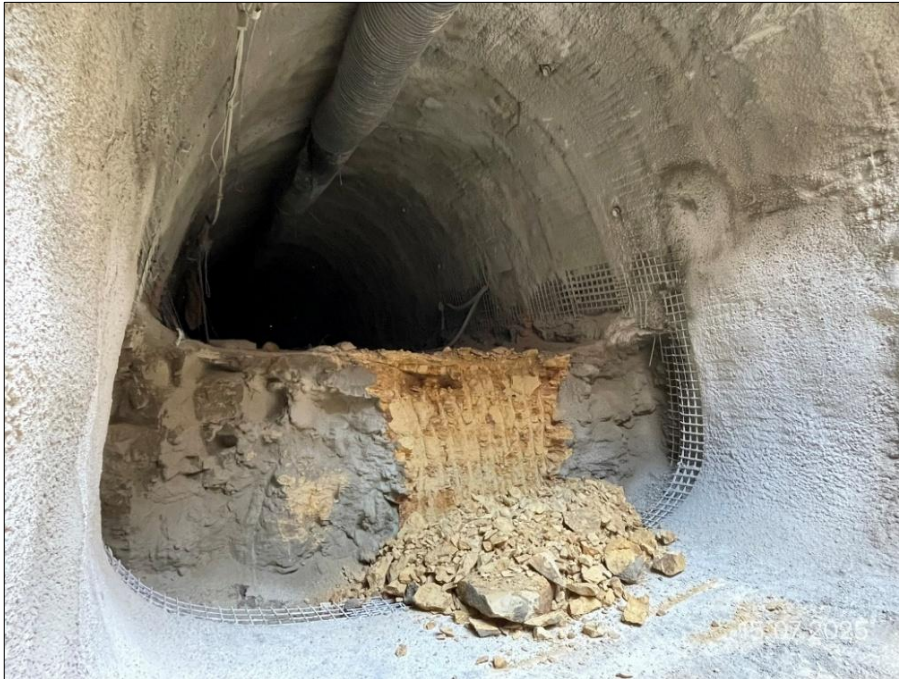
Fig. 7 Excavation of the core of the utility tunnel from the Š8 shaft towards the TK7 technical chamber (photo by the author)
