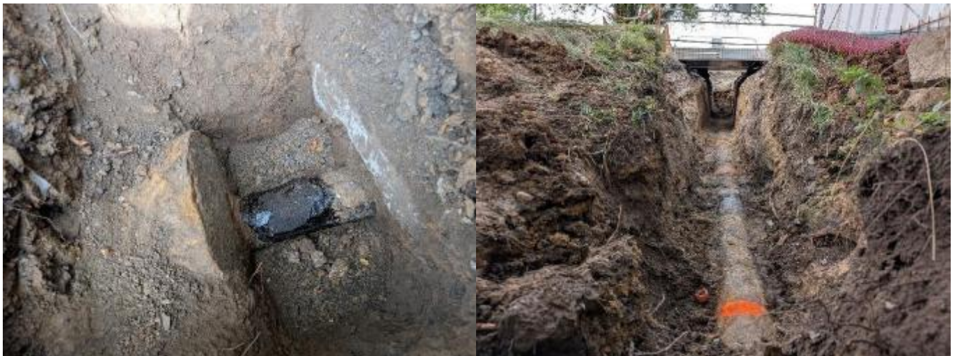
Figure 17 High-pressure gas pipeline (left), exposed pipeline (right)
