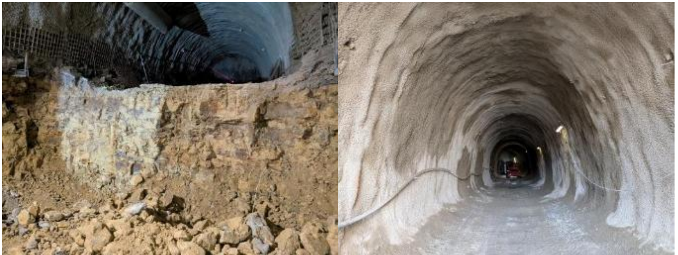
Figure 12 Core and invert face consisting of horizontal marlstone slabs (left), completed section of primary lining after profiling (right)
