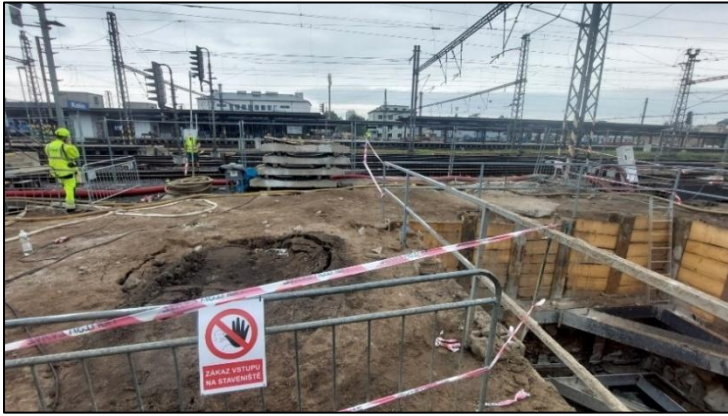
Figure 5: Surface subsidence at the launch shaft.
