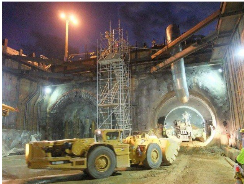
Figure 6 - Construction of Tyson Corner Tunnel, part of the Silver Line in Washington
