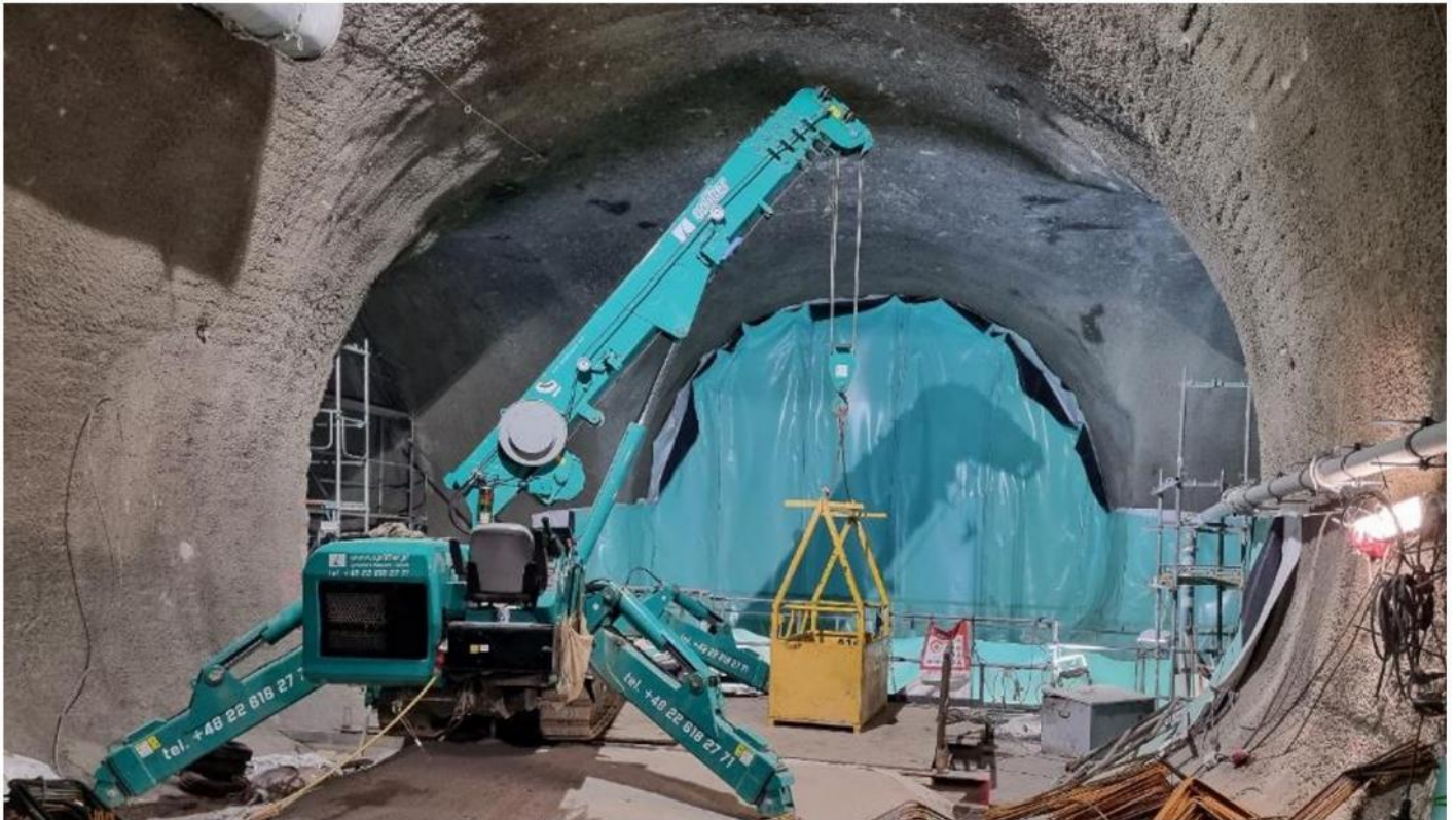
Figure 6: Special lifting equipment for operating the shafts
