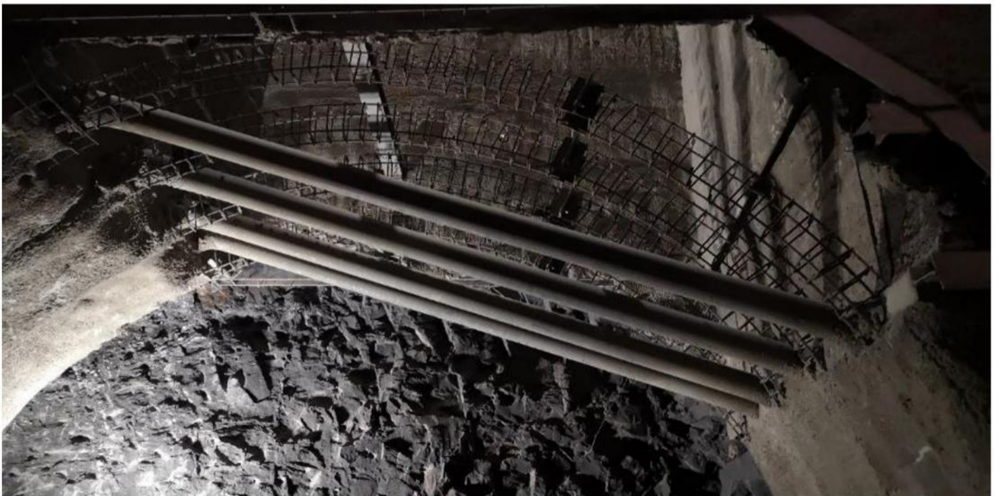
Figure 5: Spacers in the lower part of the shafts at platform level, transition to the vertical corridor
