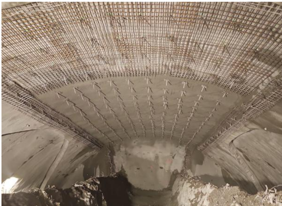
Fig. 10: Thickened station lining
