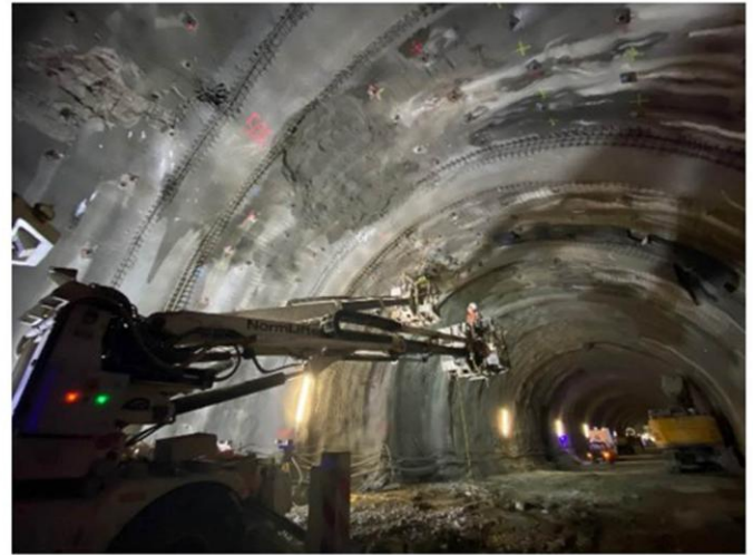
Figure 10: Crack spreading in the top heading area
