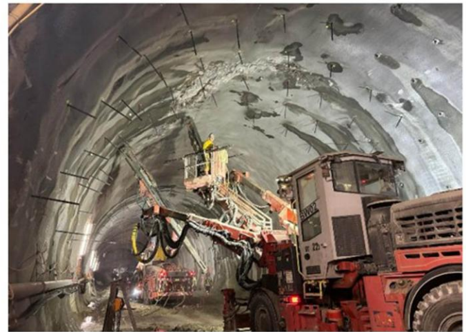
Figure 11: Anchoring after the crack appears
