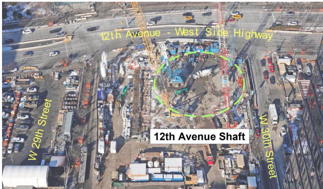
Figure 5. The 12 th Avenue shaft under construction (photo courtesy of the Gateway Development Commission).
