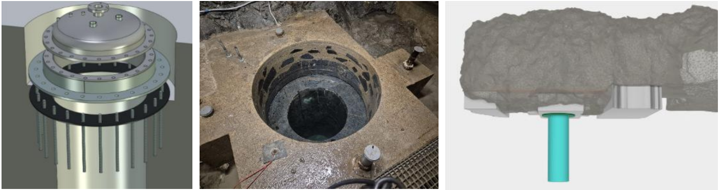
Figure 5 - Pressure seal of the rock reservoir. The reservoir will be used to monitor the behaviour of the underground system when using a liquid medium. In the centre, there is a prepared borehole with a diameter of 750 mm and a re-drilling of 1200 mm for the installation of the pressure seal, and on the right is the output from the prepared digital model of the experiment. (SVOBODA, Jiri, Lucie HAUSMANNOVA, Radek VAŠÍČEK, et al. 2016).
