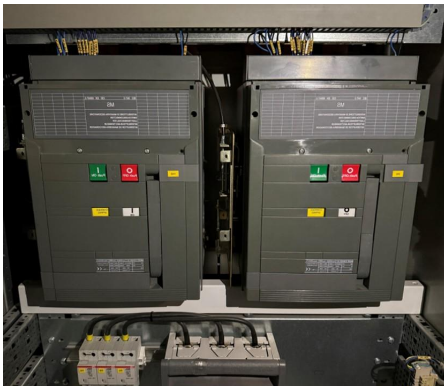
Figure 7: Power circuit breakers (deons) in withdrawable design
