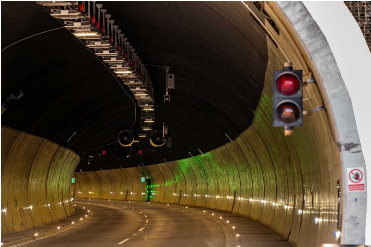
Figure 6: Tunnel tube with inductive guidance lighting
