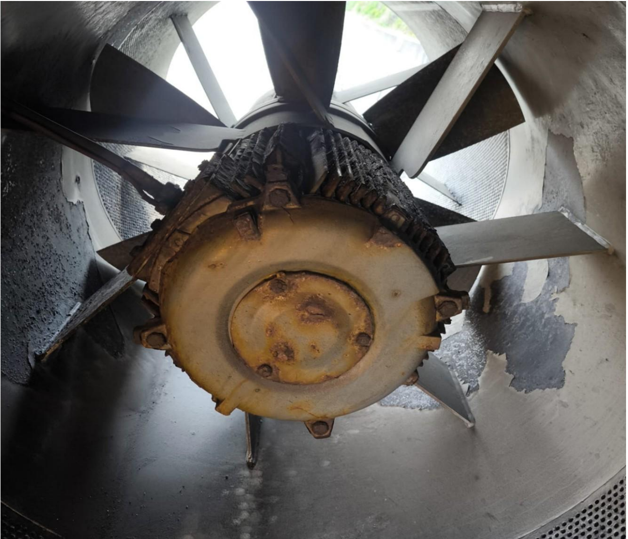
Figure 9: Condition of the original jet fans after nearly 19 years of operation
