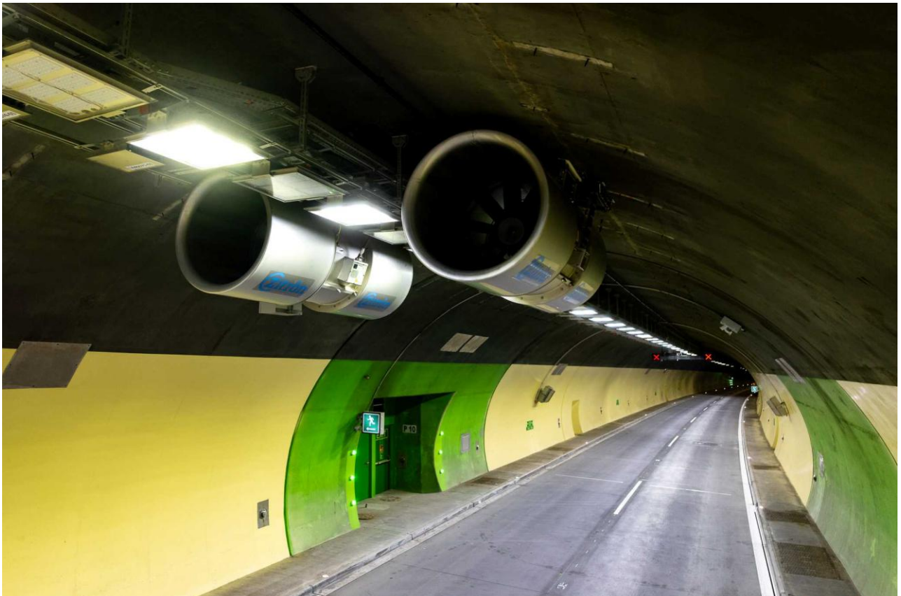
Figure 11: Newly installed ZITRON jet fans
