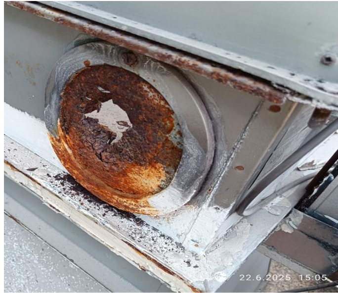
Figure 12: Condition of cross-passage ventilation equipment after nearly 19 years
