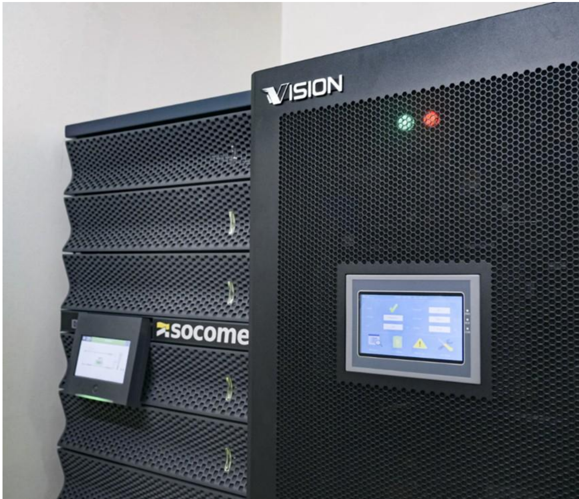
Figure 8: New UPS with Li-Ion batteries
