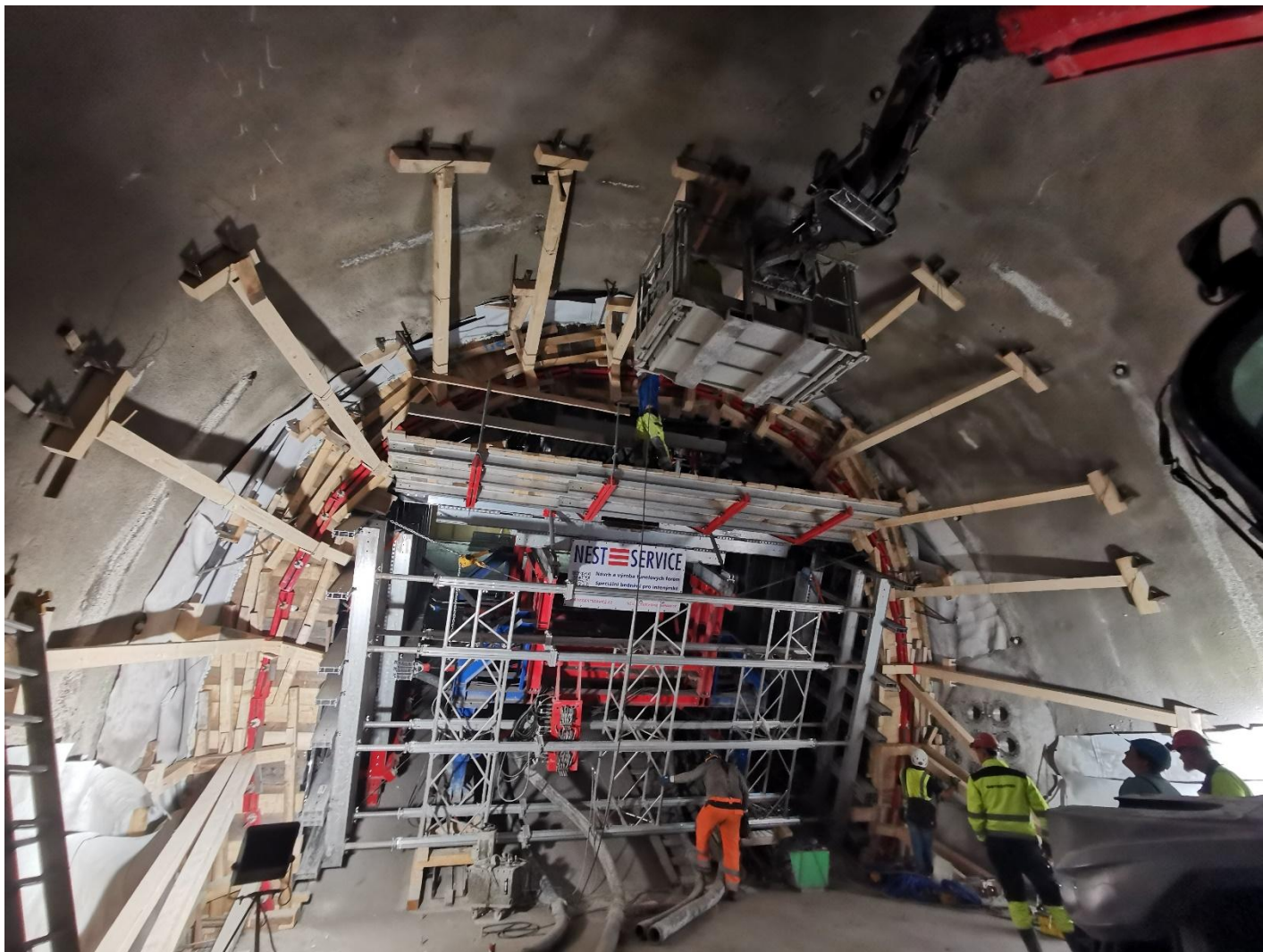
“Fig. 6 – Formwork of the first block of the upper arch of the escalator tunnel”
