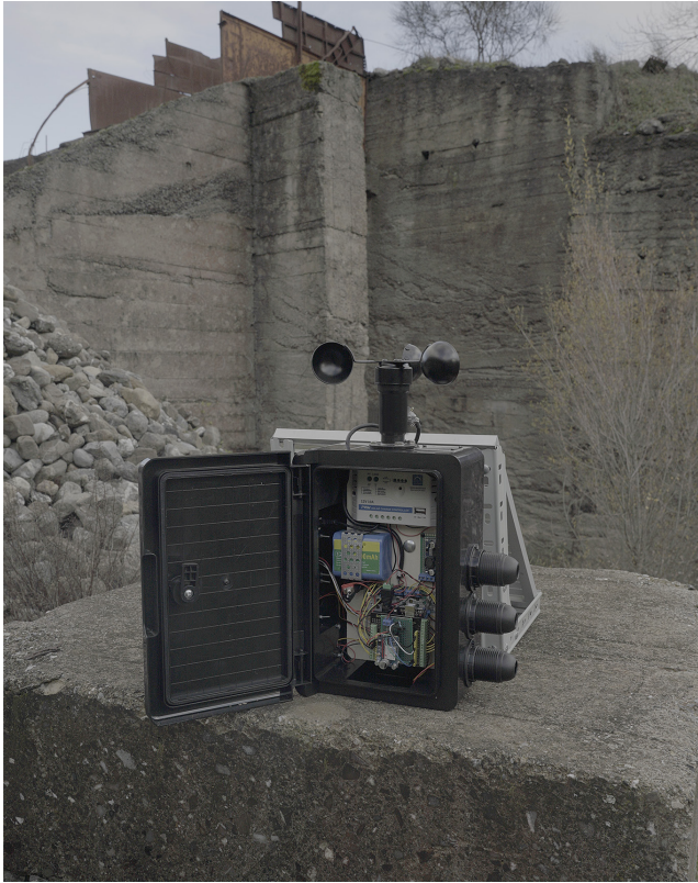
Figure 9: Residua: A Long Term Brownfield Monitoring System Oriented to Real-Time Data Sculpting in Latronico ©Carlo Gioia
