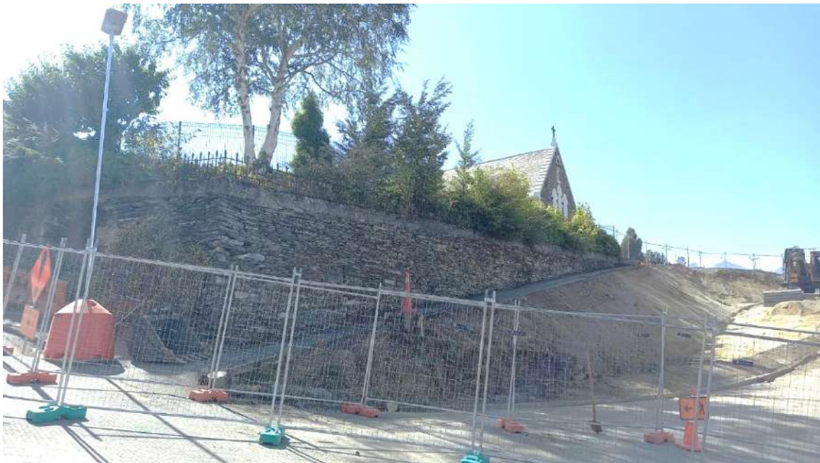
Figure 1. Original dry stacked stone wall in front of St Josephs Church at the commencement of works.
