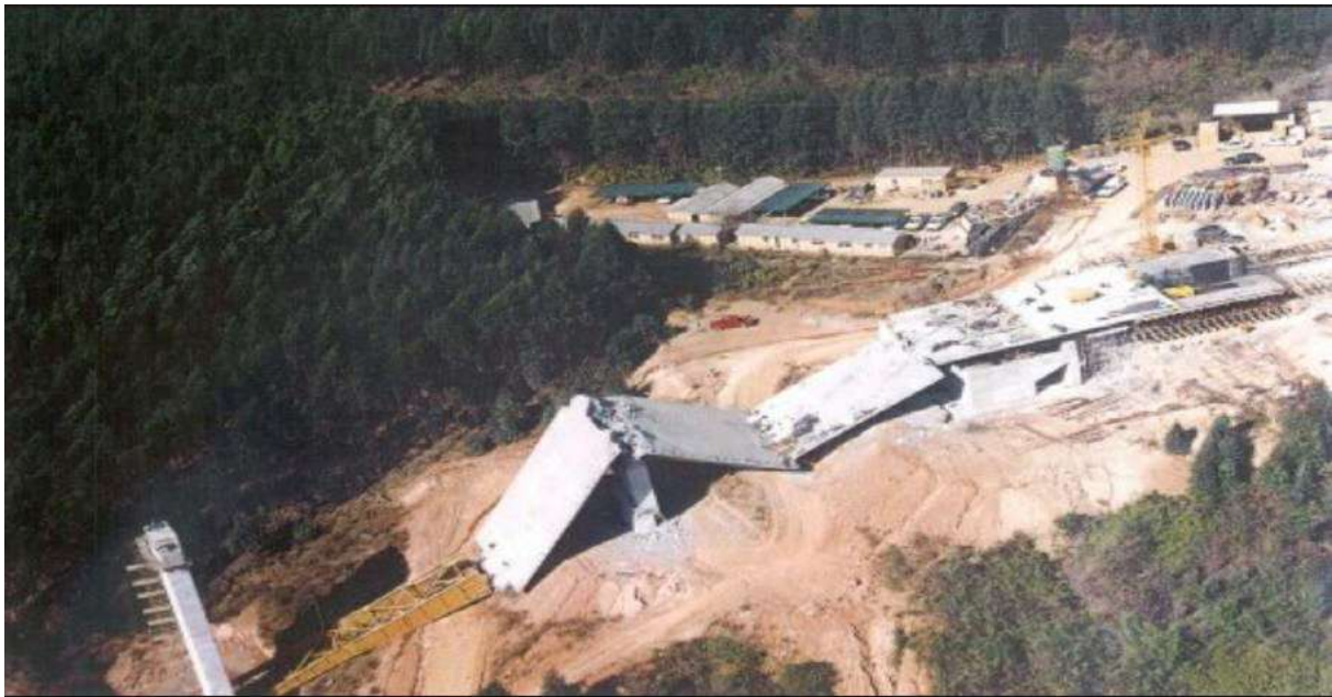
Injaka Bridge South Africa after collapsing during launching.
