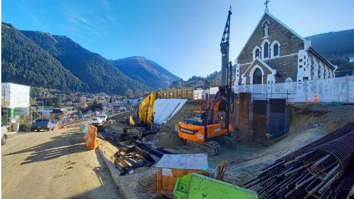
Figure 7. Piling rig and temporary retaining wall in front of the St Josephs Church, illustrating the proximity of the works to the heritage listed structure.
