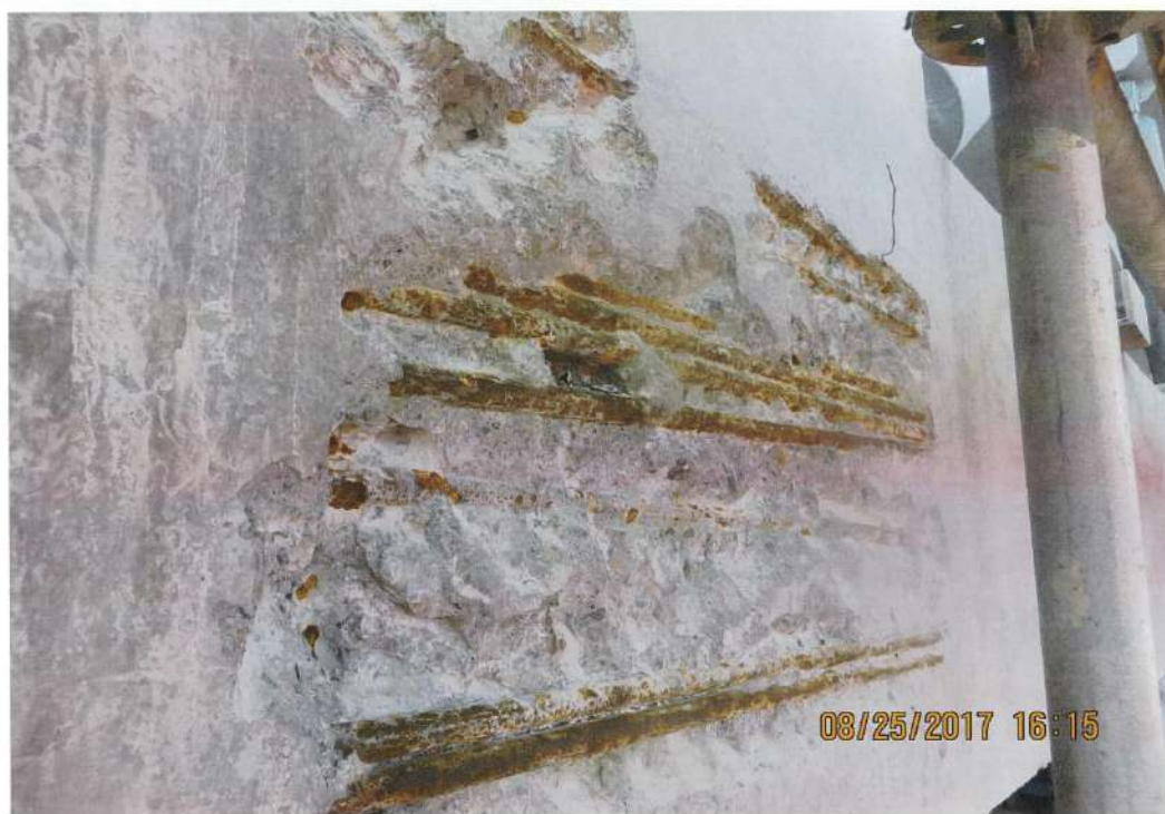
Beam Column Joint with almost zero cover when 30mm minimum specified.
