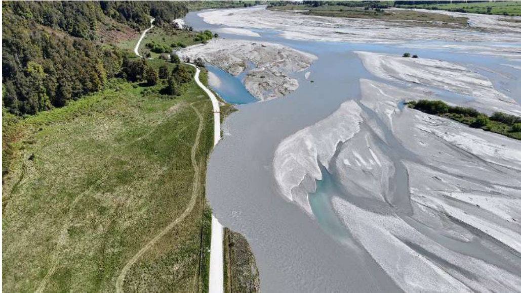
Figure 19: Erosion damage to Kinloch Road on the right bank of the Dart River (November 2024), this damage was repaired by realigning a short section of the roadway slightly inland from the river channel.
