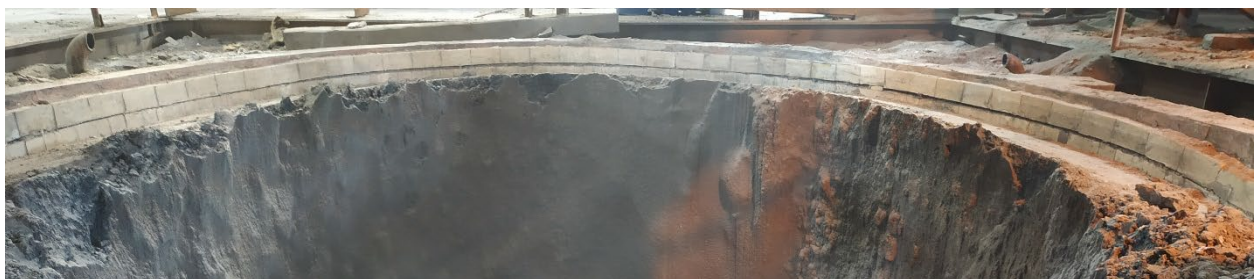
Figure 2 - Lead ISASMELT™ Furnace side wall bricks, exposed mid-campaign, showing widespread spinel coating (Hogg et al. 2018)
