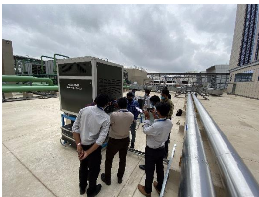
Fig.1.3: MEGHDOOT Pilot Project in Amazon Hyderabad Campus
