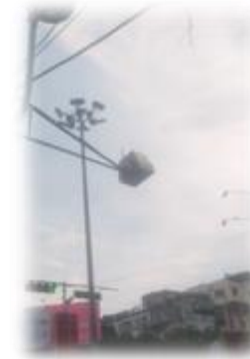
160 Street Sensors For Inundation Level
