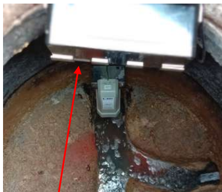
SewerEye IoT Device inside the Manhole Chamber
