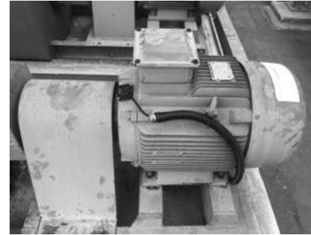
Pump condition monitoring
