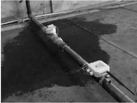
Water meter / flow monitoring
