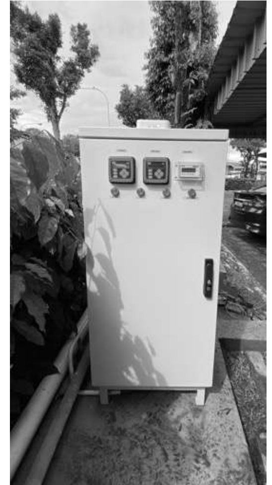
Water Skid Process monitoring / control
