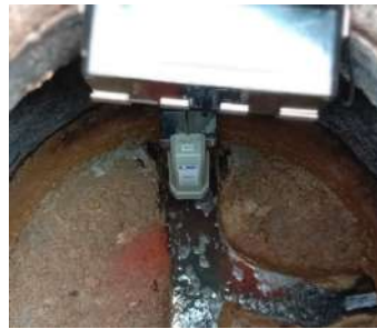
Level / Flow Monitoring at Sewer Manholes
