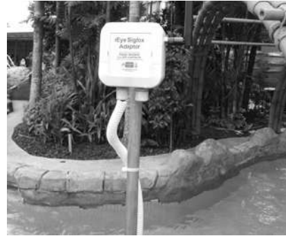
Water leak detection
