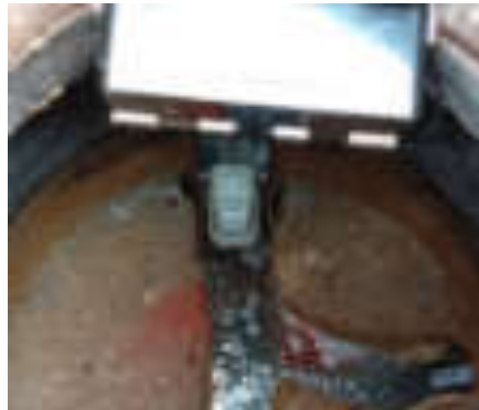
Level / Flow Monitoring at Sewer Manholes
