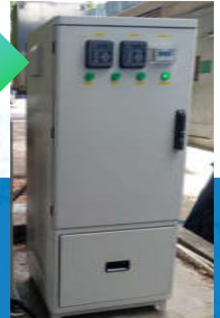
Standalone commercial I2BioS installed in a factory located in Singapore (R) (2018)
