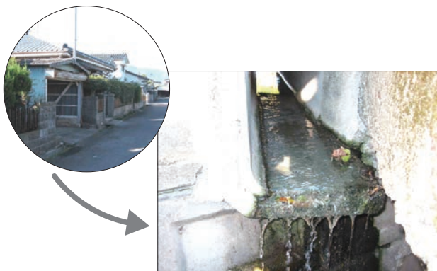
A road gully in tandoku-shori Johakasou installation area in 1970s (where whitish sludge was attached to)
