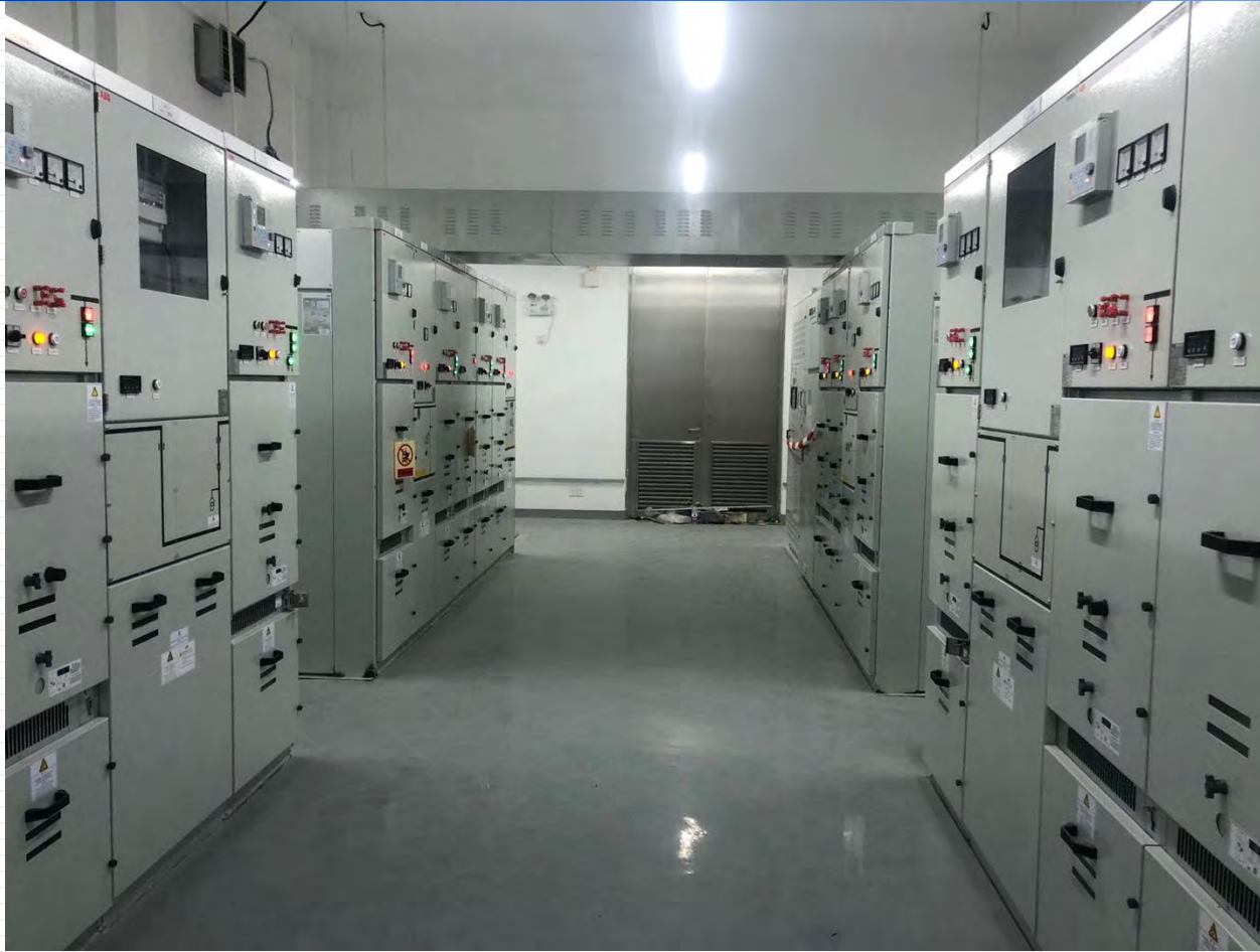
Shore-based power supply and transformation equipment
