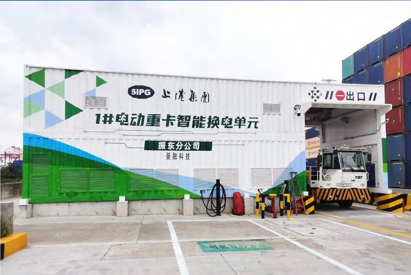
Power swap station for internal container truck
